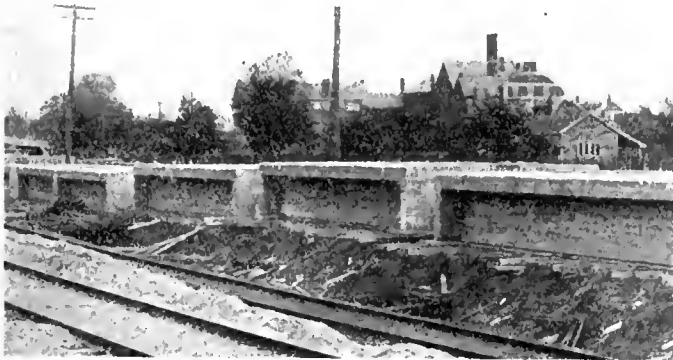
These girders will compose the deck of the concrete trestle bridges on the Leaside-North Toronto C.P.R. line.
